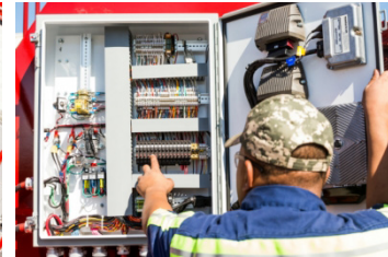
Easy Access to Heavy Duty Circuit Breaker Panel and Breaker Reset Switches
